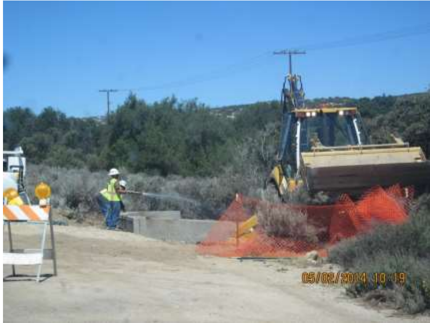
Photo 5: In accordance with MM-BIO4-A and MM-AQ-1, water trucks equipped with hoses are utilized to control dust in areas of active construction.
