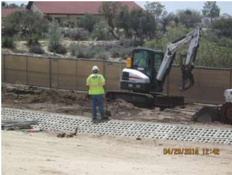
Photo 6: In accordance with MM-VIS-3c, opaque visual screen fencing was routinely maintained at the Boulevard Substation.
