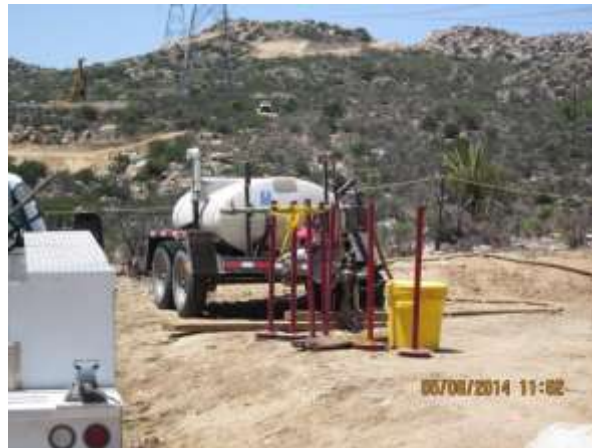
Photo 4: Drip pan containment bins is placed beneath equipment staged along the right-of-way in accordance with MM-HAZ-1a and spill kits were accessible in case of hazardous materials leak.
